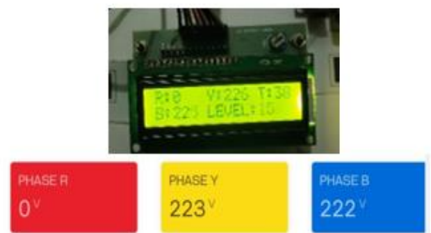
Figure 13 Open Circuit Fault in R-Phase
