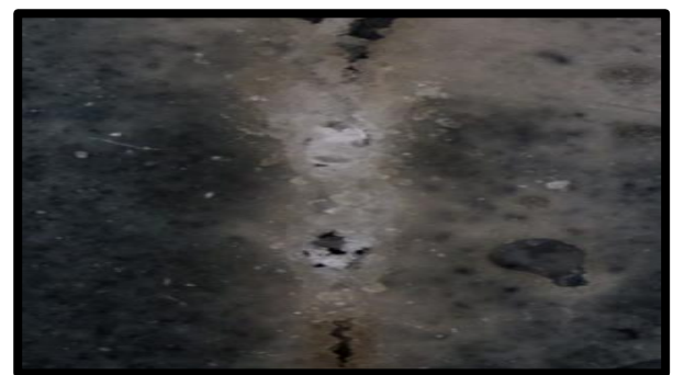
Figure 7 Calcite Formation on Cracks
