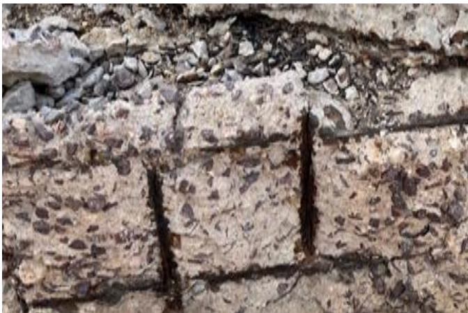
Figure 3 Shows the Reinforcement Visible in the Stair After the Concrete Fire
